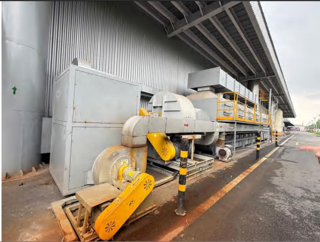
“干式高效除雾过滤+活性炭吸附+脱附+催化燃烧”设备
